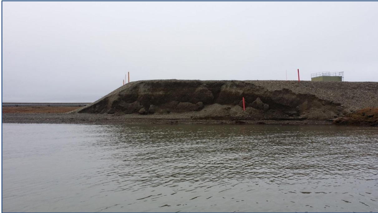
Figure 4-7. Photograph of Site 2 – WEST Showing Erosion of AGI Pad
